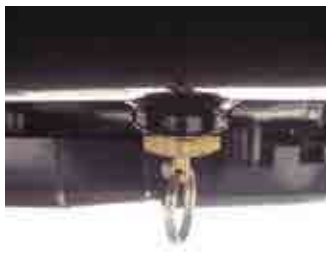
Tank water draining valve
